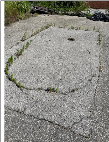
Lot patch left side of rear lot. Unclear what cause for patch was, possible old UST
