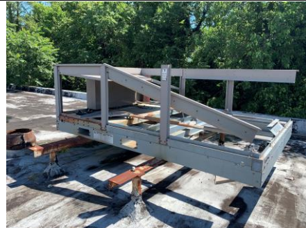
Rooftop equipment (AC compressors/air handlers), previously removed
