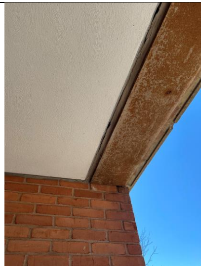
Grey caulking at entryway ceilings, positive for asbestos
