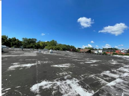
Multi-layer asphalt roofing including asbestos containing roofing felt, black tar and black flashing cement
