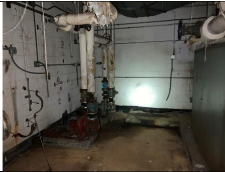
White end cap mastic and canvas wrap are present throughout the boiler room, and run throughout the building above the ceilings and in chase walls
