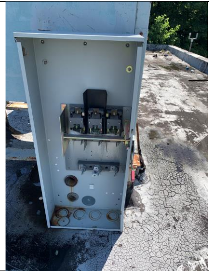
Rooftop equipment (AC compressors/air handlers), previously removed
