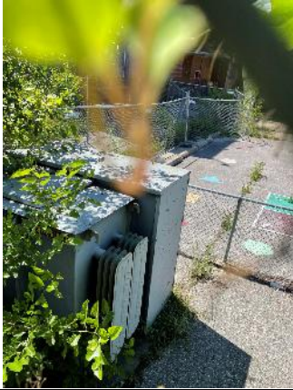
Large transformer located at north edge of property
