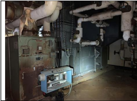
Boiler system is fiberglass jacketed, canvas pipe wrap and white end cap mastic are positive
